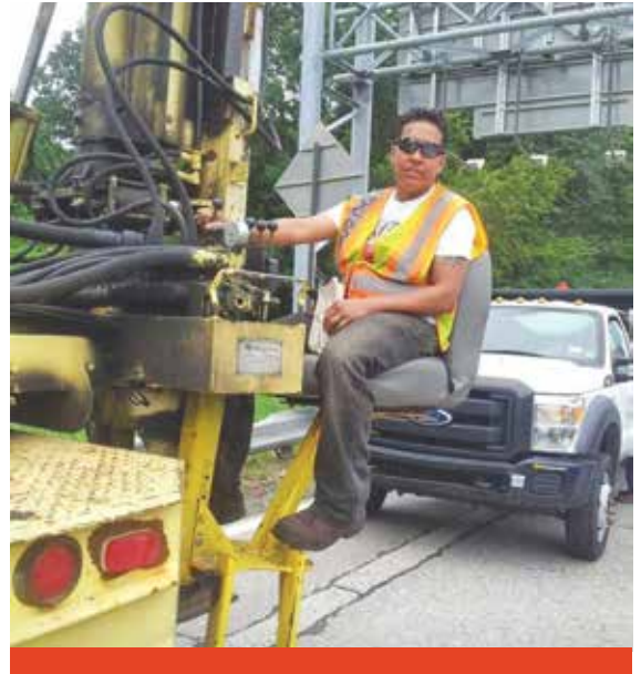
Sharon Massa works the pounder as a Department of Transportation Assistant City Highway Repairer at Kew Loop Yard in Queens. The post pounder is used to remove and install posts that hold up highway guardrails. Massa is one of the less than 5% of women who operate this machine.
